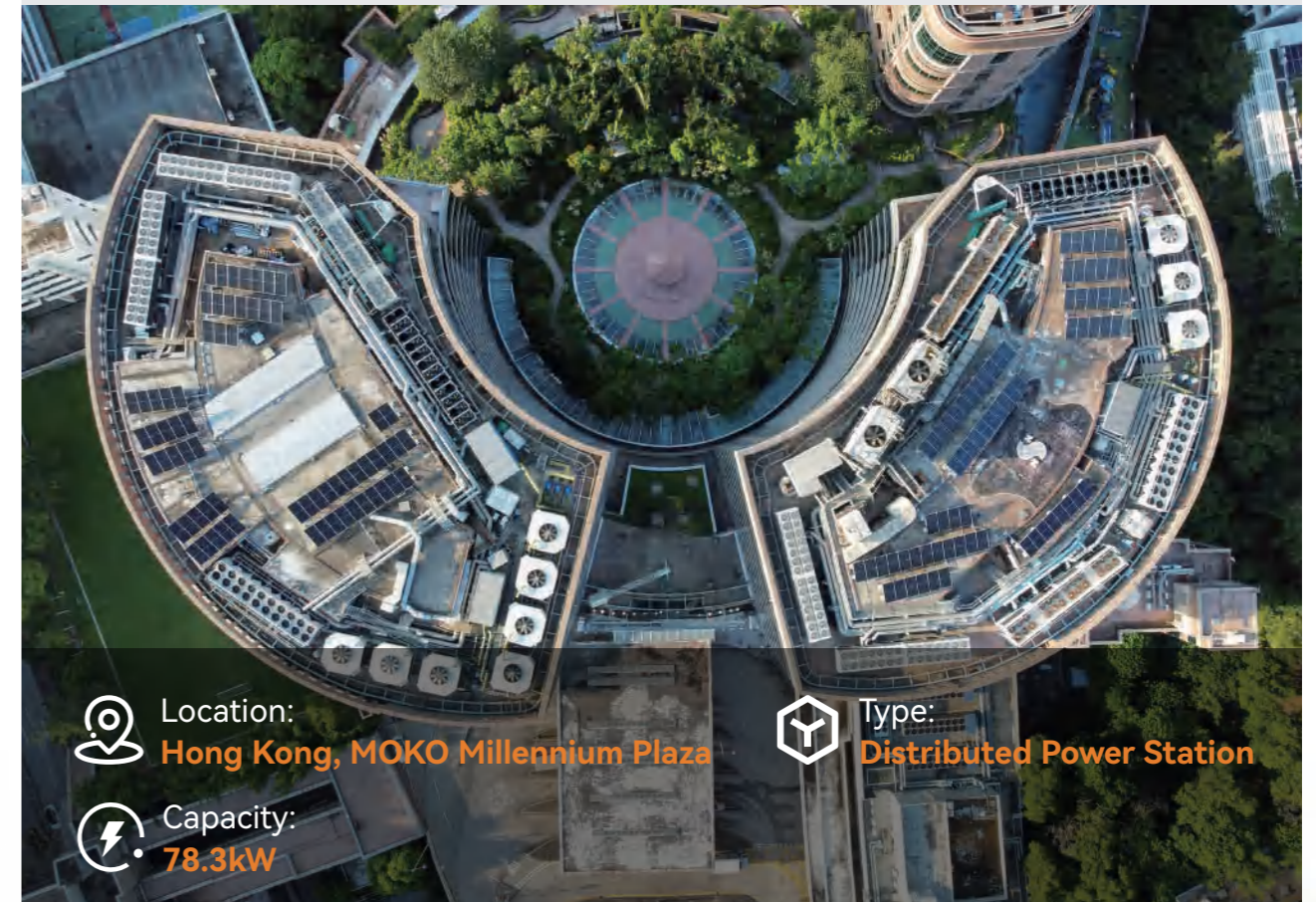
MOKO Plaza, Hong Kong | 78.3kW Distributed Power Station Products: Bifacial Module 415W (2023)
