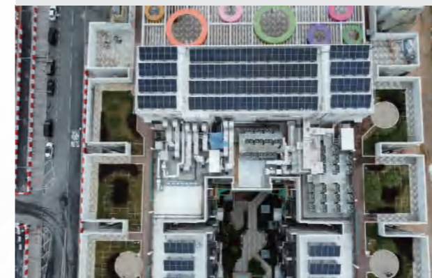
Kwu Tung, Hong Kong (2023) 78.3kW Distributed Power Station
